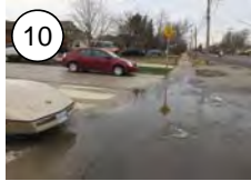
10 OPPORTUNITY Improve drainage
