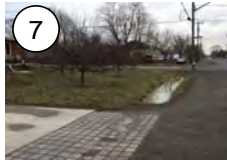
7 OPPORTUNITY Improve drainage
