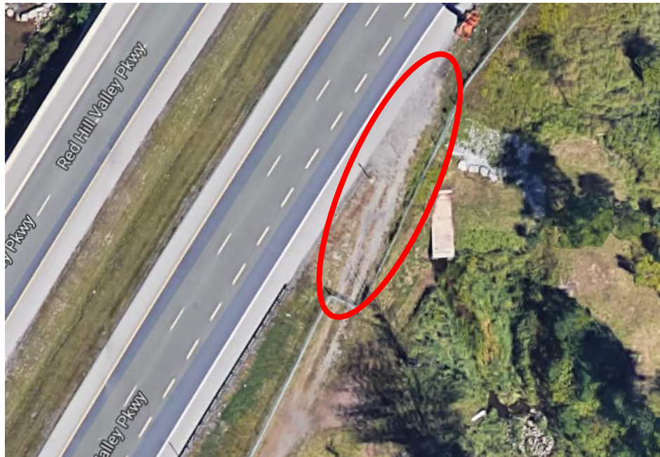
Figure 31: Unpaved Access North of Greenhill Avenue
