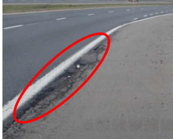
Figure 29: Pavement Edge Drop-off
